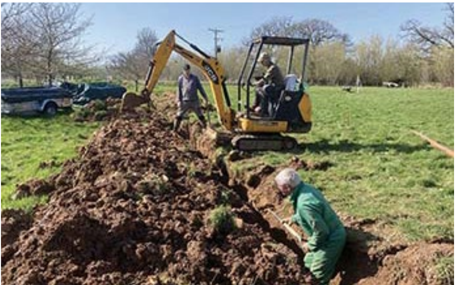
Installing the pipe which will take the outfall from the tunnel drainage pumps. Pete Clark is driving, Neil Evans is digging and Chris Kelly is checking the alignment. Photo by David Hartland.
