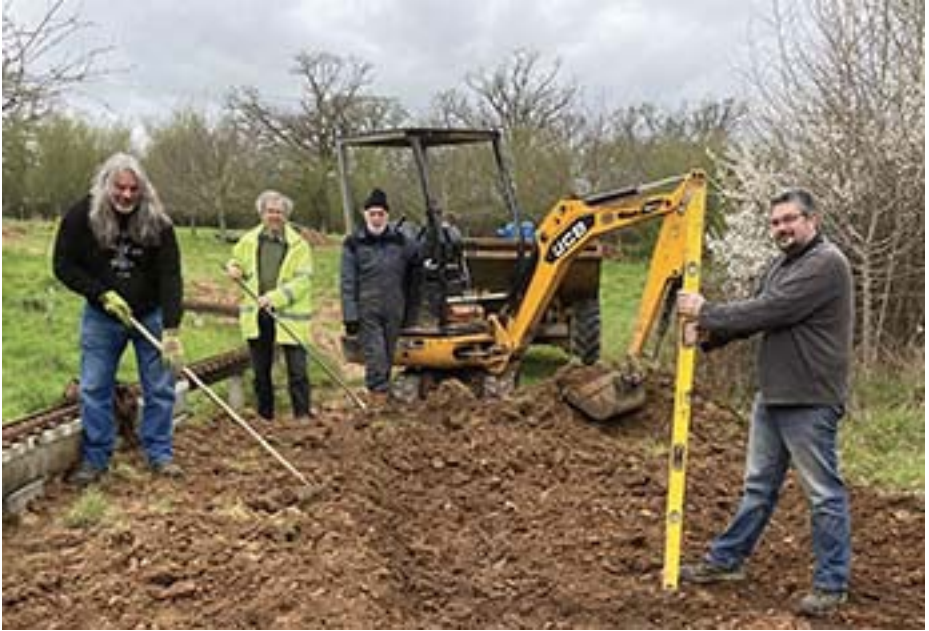
Breaking ground on the Yonder Field project – Dell Warren, Steve Gosling, Barry Baxter and Adam Farrance. Photo by digger driver David Hartland.
